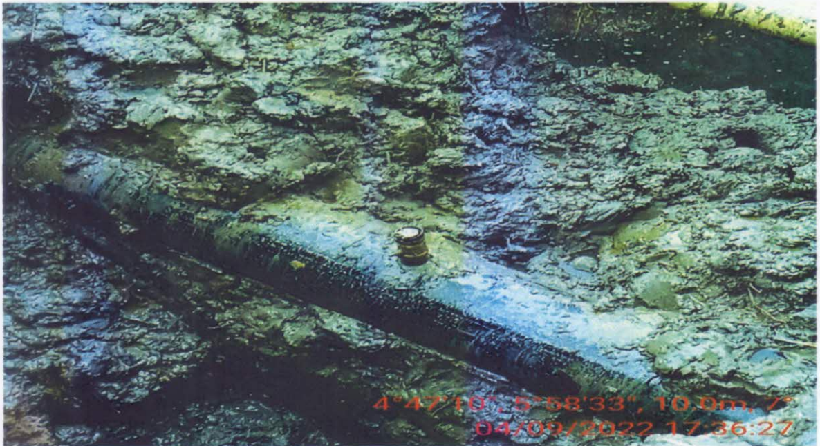
PICTURE 1: SHOWING 2" VALVE INSTALLED ON THE PIPELINE FOR OIL THEFT
